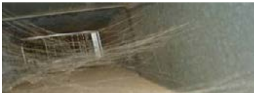
Figure 2. Presence of insects in the air ducts. 9
