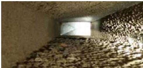
Figure 1. Air duct accumulated with dust. 9
