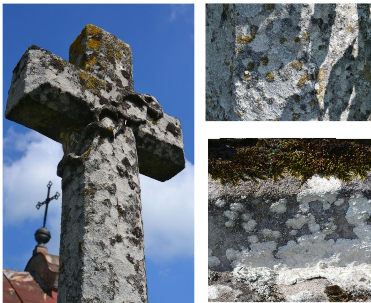
Fig. 1. Biogrowths and the destruction of stone caused by them on the cross from the cemetery in Pidkamen
