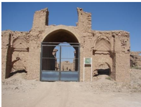
Fig 7 Entrance gateway of the Stone Caravanserai of Mohammadabad (source: Cultural Heritage Organization of Qom)
